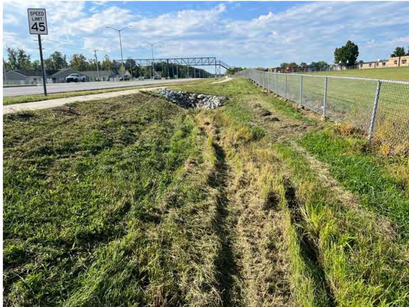
Photo 1. Looking south at roadside culvert inlet and beyond the southern investigated area extent.
