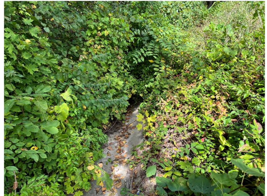
Photo 24. Looking northwest at concrete lined roadside ditch and herbaceous vegetation along the west side of North Clinton Street.
