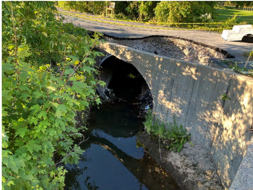
Photo 83. Looking northeast at the small structure that conveys Swift Ditch under Clinton Street.
