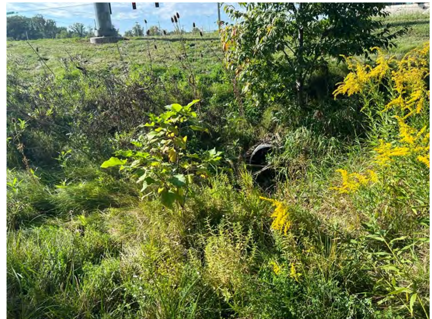
Photo 8. Looking south at roadside culvert inlet and herbaceous vegetation along the west side of North Clinton Street.
