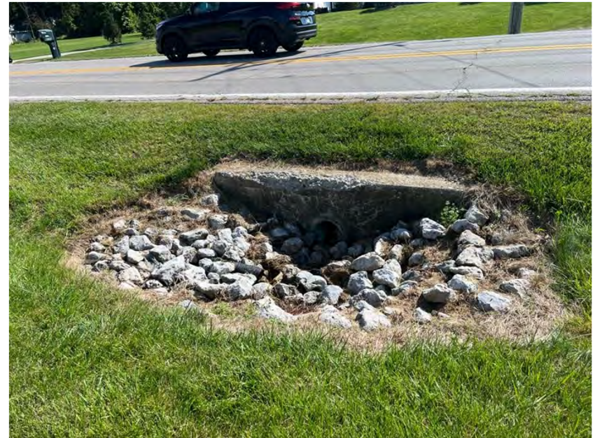
Photo 56. Looking east at small structure inlet with riprap and maintained grassy ROW.
