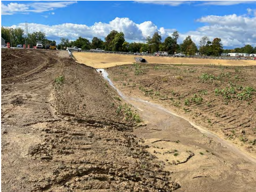
Photo 137. Looking southwest at bare ground under construction and a dry bottom retention pond.
