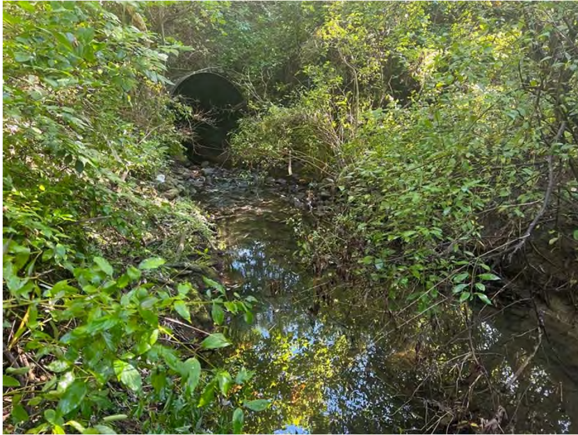
Photo 85. Looking downstream (south) at Swift Ditch and the small structure that conveys the stream under Wallen Road.
