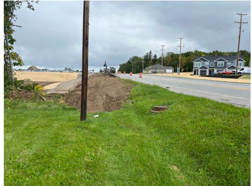
Photo 134. Looking northeast at maintained grassy ROW and bare ground along the west side of North Clinton Street.
